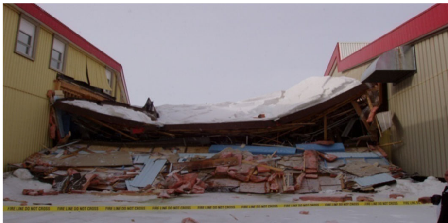
2004, foyer roof collapsed of Samuel Hearne Secondary School in Inuvik
